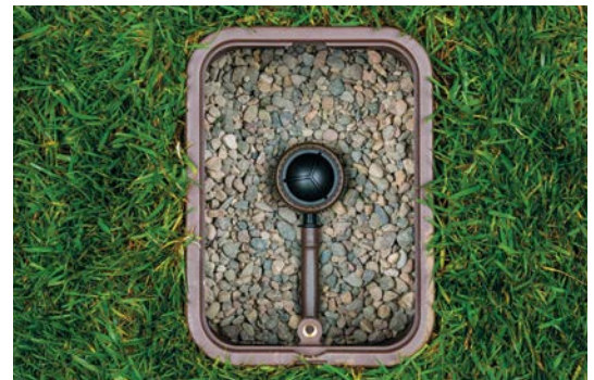
Automatic Flush Valve Installed
