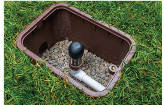
Air/Vacuum Relief Valve Installed
