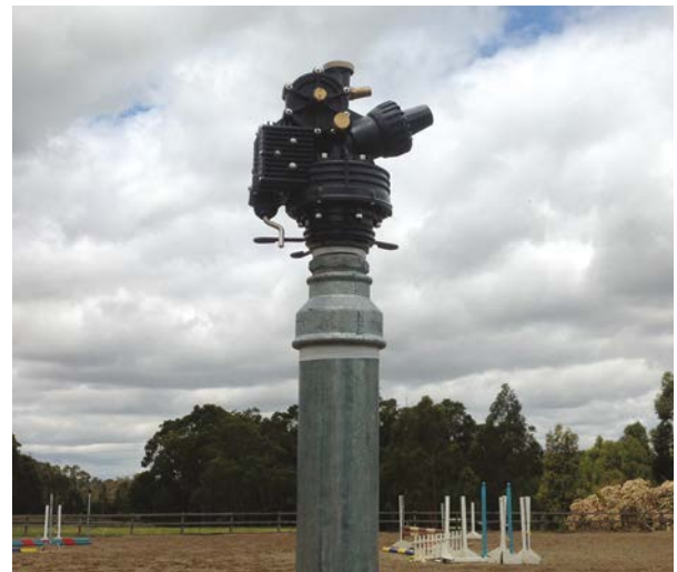
ST-1600-HS-BR Rotor Installed
