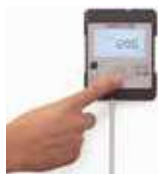
HMI control system on wall
