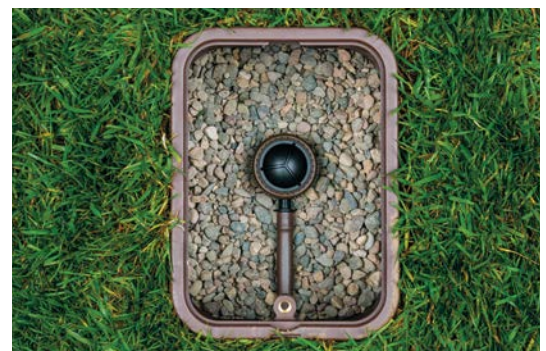
Automatic Flush Valve Installed
